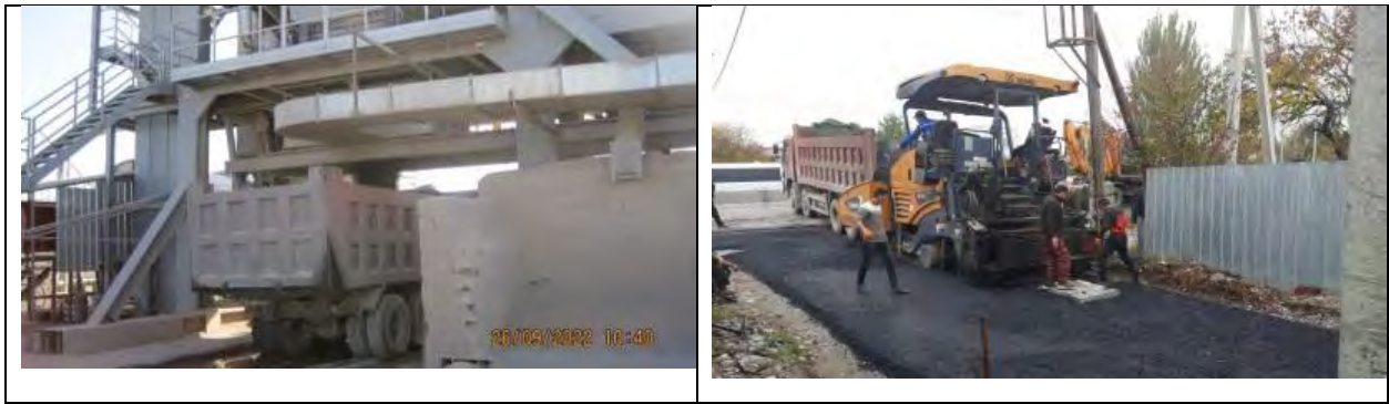
Figure 33 Loading of asphalt mixture into dump trucks and unloading into asphalt pavers
