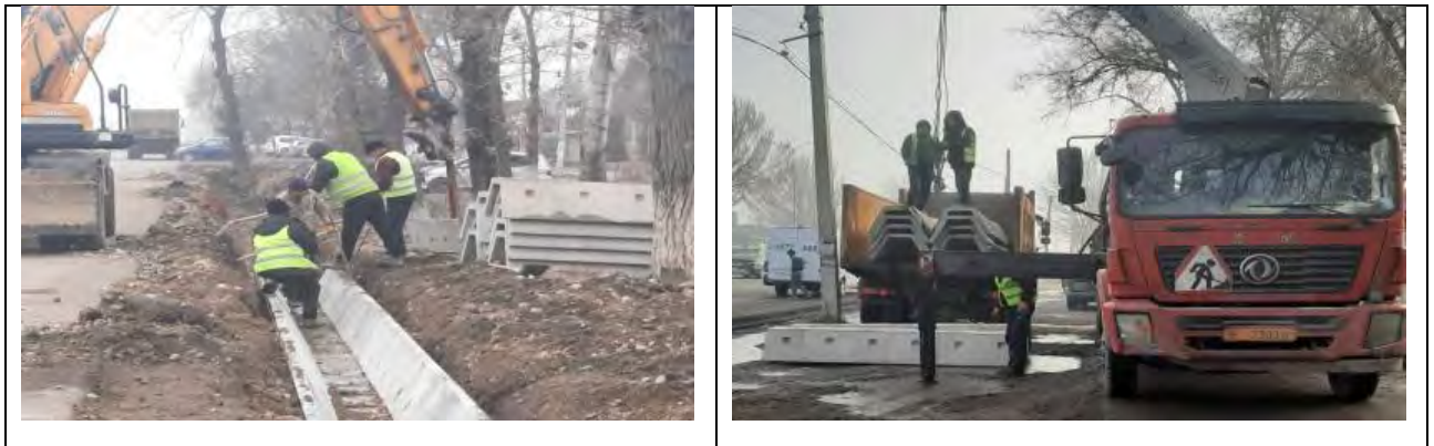
Figure 67 Failure to comply with safety precautions when moving load with a crane
