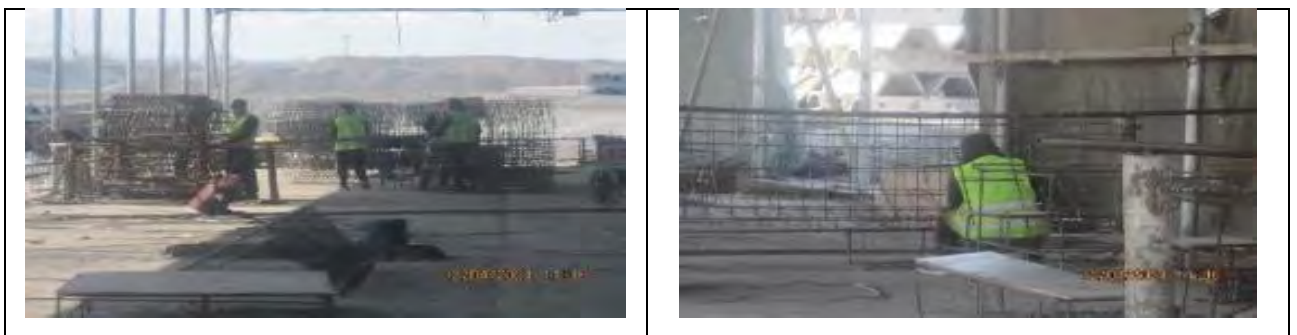
Figure 47 Production of reinforcing welded meshes, frames for the production of reinforced concrete structures
