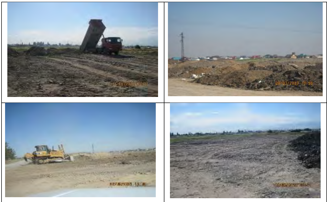
Figure 64 Storage and levelling of unsuitable soil for further use in the villages of Voенno-Antonovka
