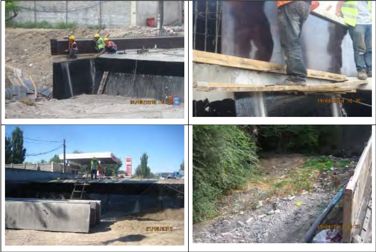
Figure 47 Safety violations during the construction of bridge on the Krepostnoy Canal
