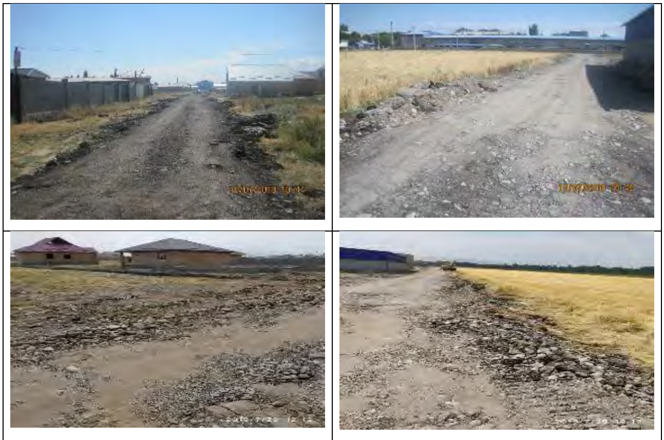
Figure 28 Taking out of old asphalt to the territory of the "Yntymak" residential area at the request of residents and representatives of the Mayor's Office of Shopokov
