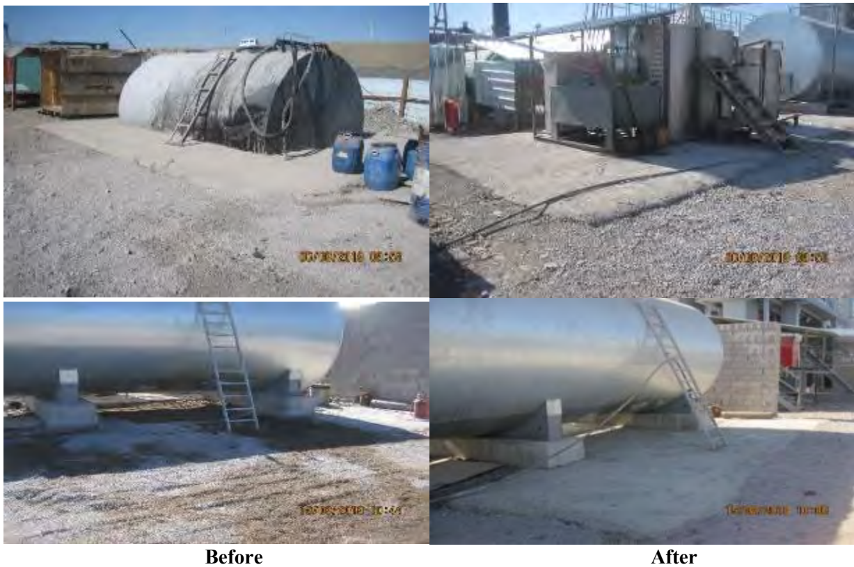
Figure 72 Impenetrable protective coating around chemical containers
