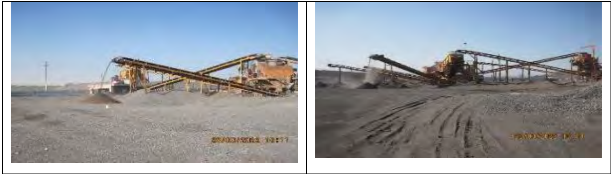
Figure 30 Stone crushing plant
