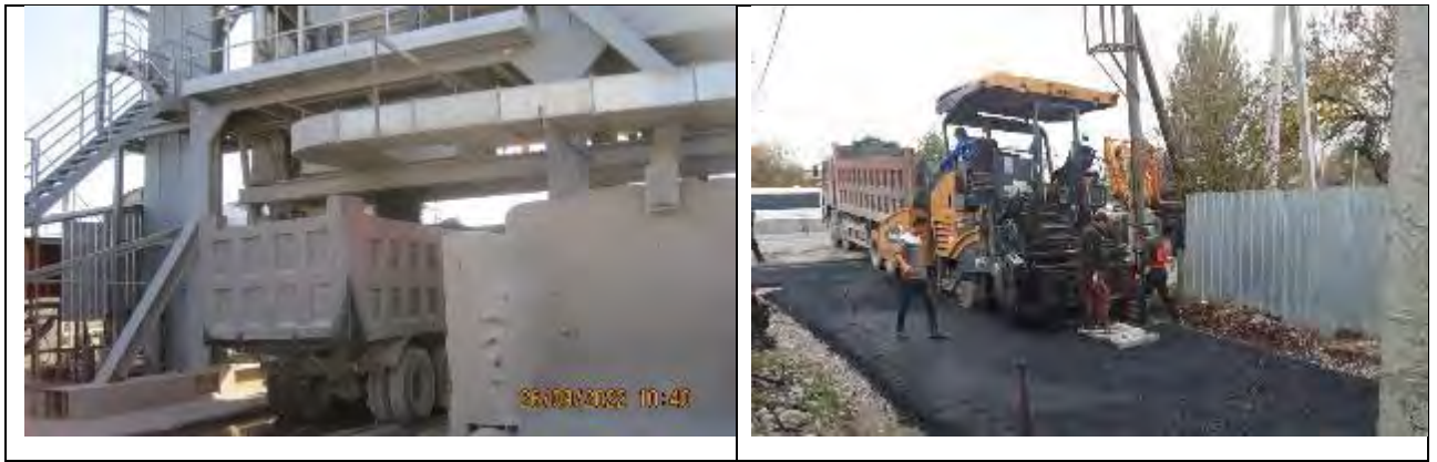
Figure 68 Loading of asphalt mixture into dump trucks and unloading into asphalt pavers
