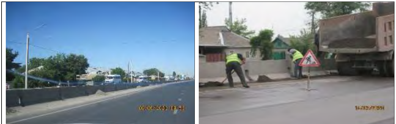
Figure 57 Cleaning of parapets from soil waste and removal of waste from the road
