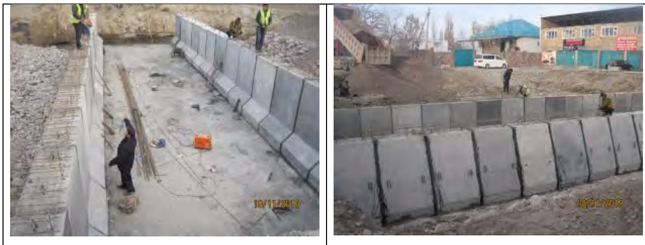
Figure 45 Safety violations during the construction of the bridge on the Jantai Canal
