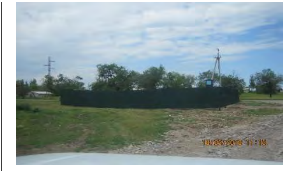
Figure 28 Rehabilitated well to supply the plant with water
