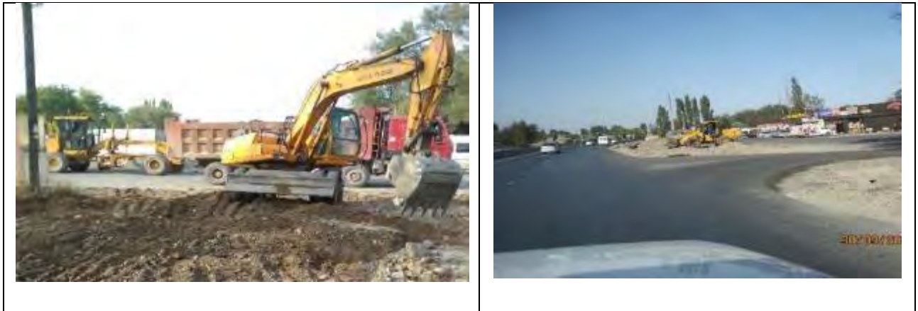
Figure 35 Laying asphalt at junctions to the streets adjacent to the road in the village of Aleksandrovka
