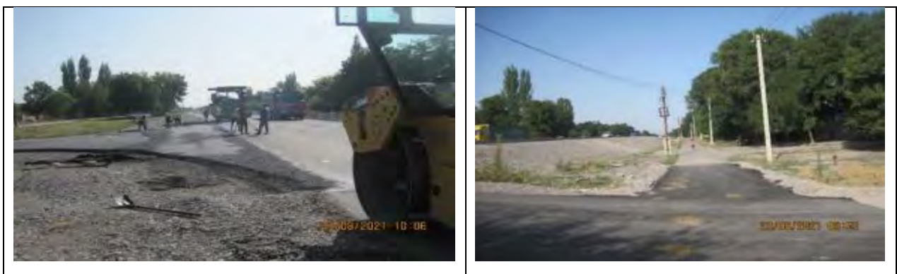
Figure 36 Laying asphalt at junctions to the streets adjacent to the road in the village of Petrovka
