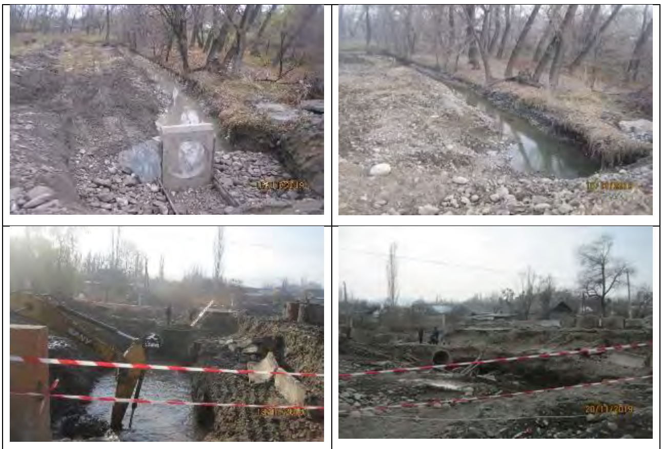
Figure 52 Wedging out of groundwater during the construction of culvert pipes
