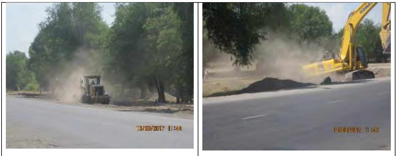
Figure 12 Dusting observed during the removal of topsoil
