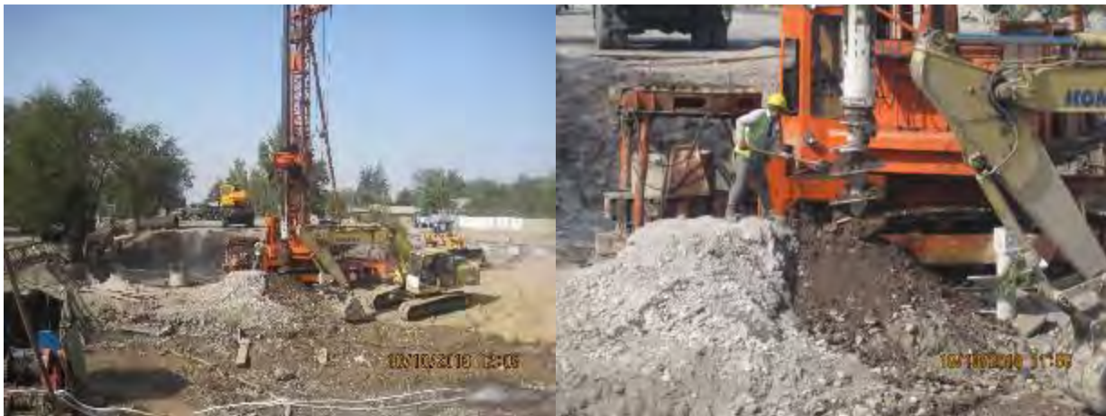
Figure 41 Construction of a bridge across the Ak-Suu river by drilling on the left bank
